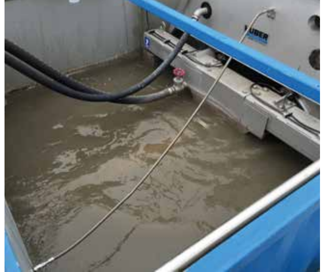
HUBER Drum Screen LIQUID for maximum separation efficiency and at the same time low pressure losses.
