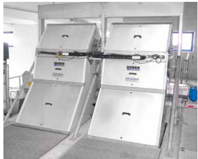
Two HUBER Fine Screen STEP SCREEN® SSF units installed in parallel channels.
