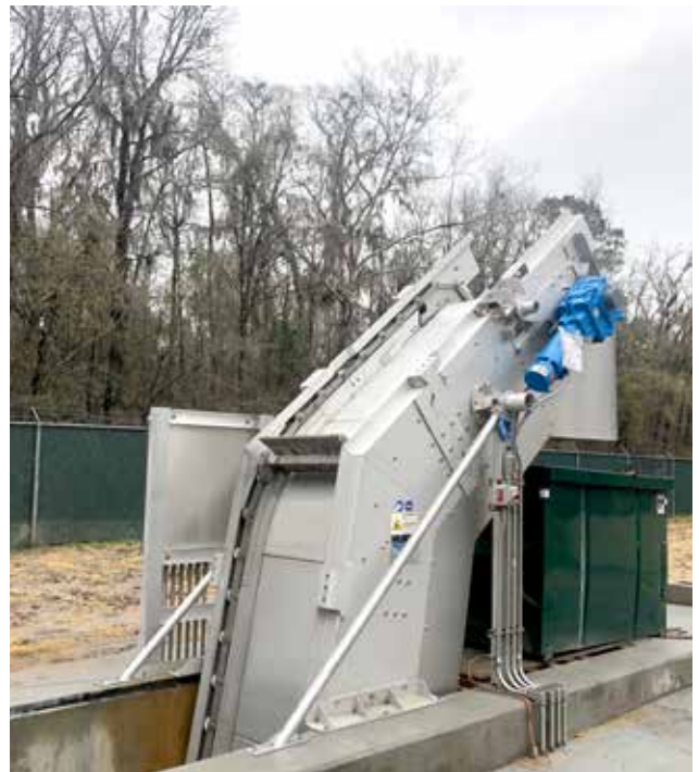
Screen installation in the inlet of a pumping station with discharge directly into a container.
