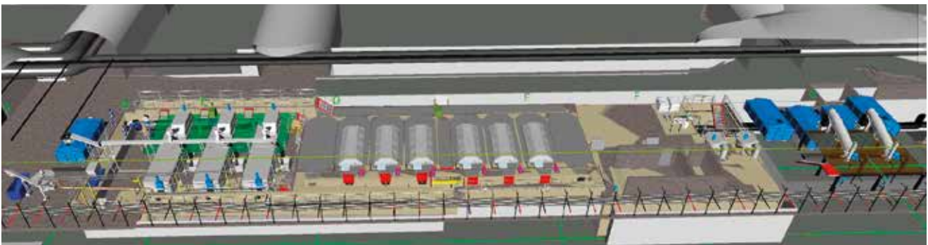
Fig. 4: River and sea outfall with 6 HUBER Drum Screen LIQUID units as replacement for a primary settling tank.
