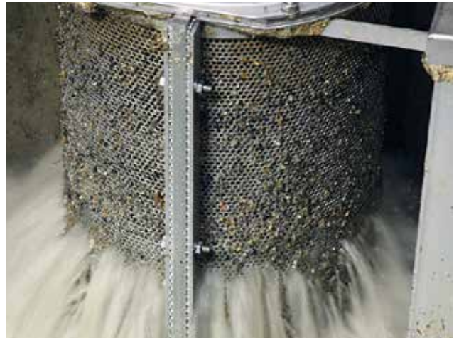
HUBER Pumping Stations Screen ROTAMAT® RoK4 in operation.
